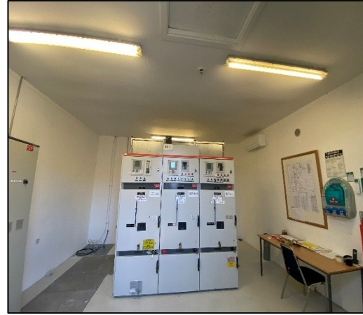
Plate 4-22 Interior of the control building.
