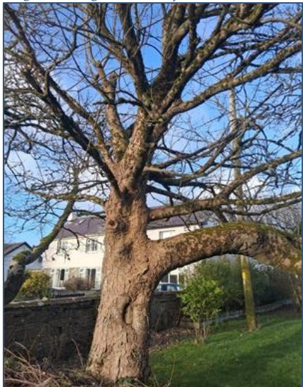
Plate 4-13 Pinch point location 18 - oak tree with superficial knot hole and tear out to be removed.
