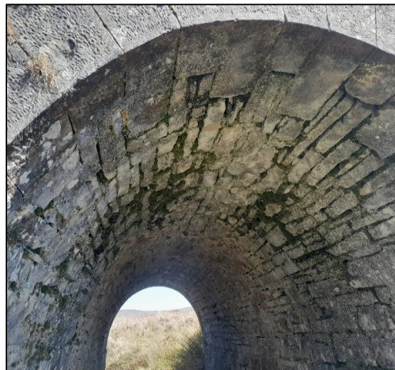
Plate 4-24 Gaps visible between the stones of Bridge 1
