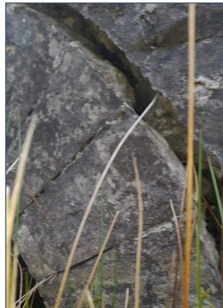
Plate 4-28 Gap in the stonework of the bridge providing roost potential for bats.
