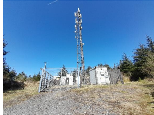
Plate 3-4 Example of operational wind farm infrastructure, comprising fenced compound and associated control equipment, assessed as having Negligible suitability for roosting bats.
