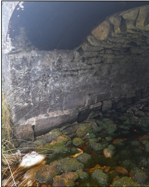
Plate 4-25 Bridge 2 with crevices visible in between the stones
