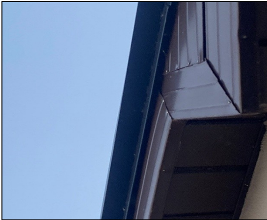
Plate 4-21 Fascia lifting along gable of control building.
